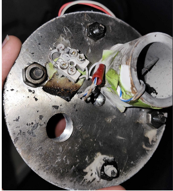
Fig. 2 Melted wire terminals after 5 gram test
